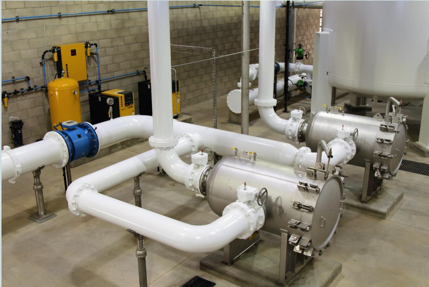
INLET PIPING AND FILTERS
