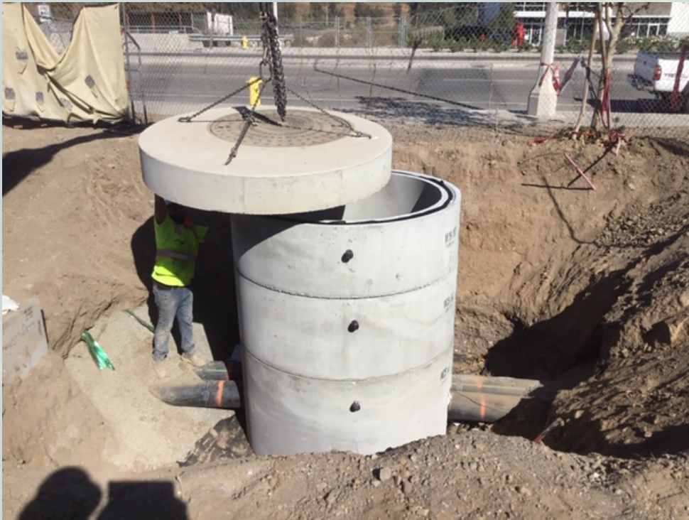
SEWER FORCE MAIN MANHOLE ( FOR SURGE VALVES)
