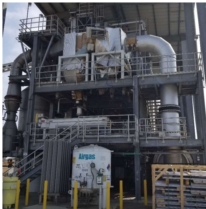
Figure 18: Biosolids Dryer at WRF No. 1
