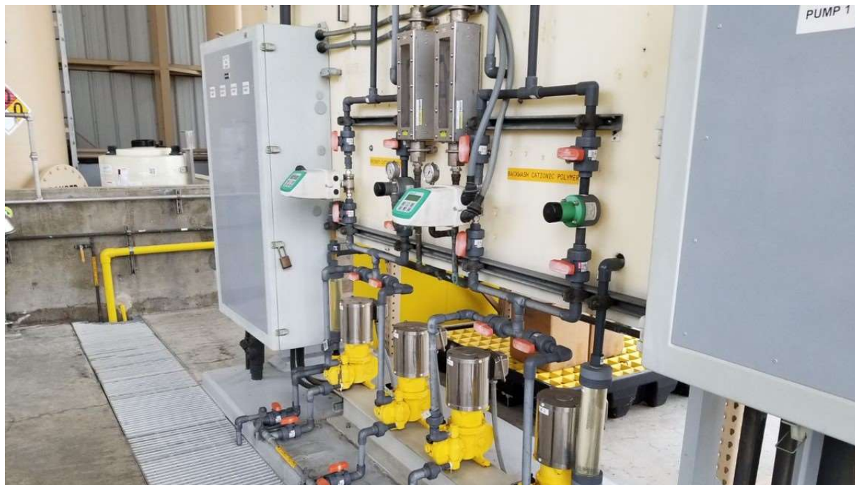
Figure 14: Chemical Pumps at Lester WTP
