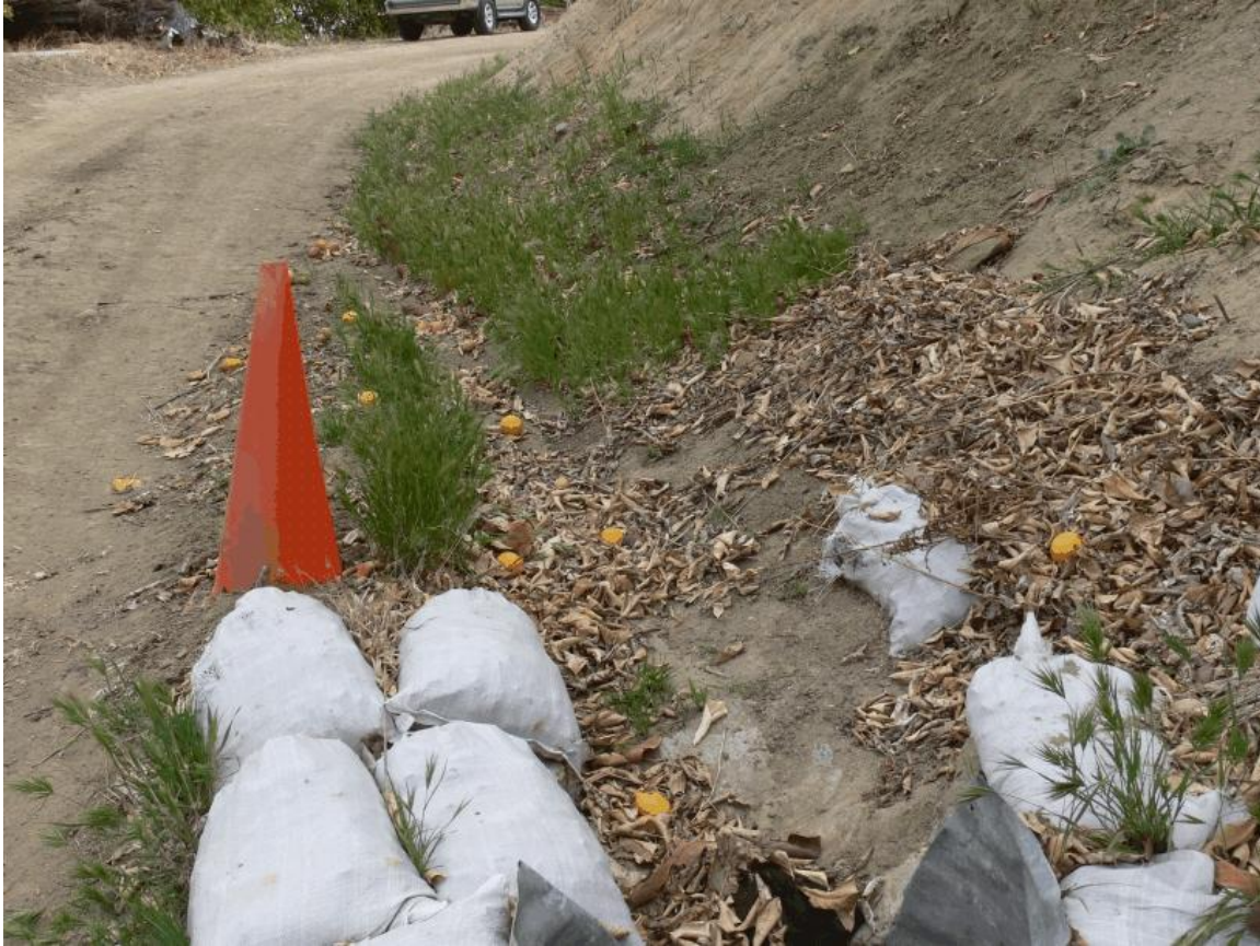
Drain A (photo 6): Head of side tributary to Drain A. Water runoff from road collected in pipe in foreground and piped down to lower road.
