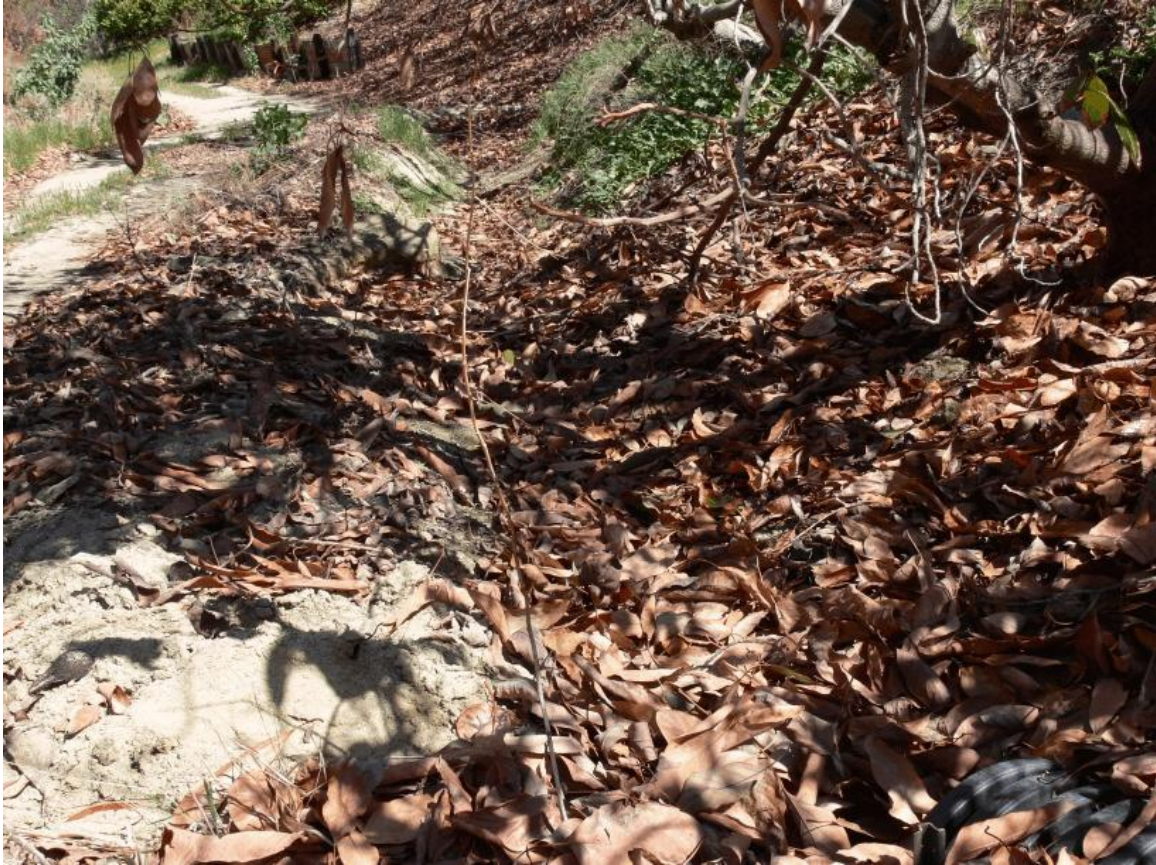
Drain A (photo 8): Drain exits from pipe in lower right corner of the photo into this leaf-filled ditch which it follows into a pipe that connects it to the main line for Drain A on the other side of the road seen in the upper left corner of this photo.
