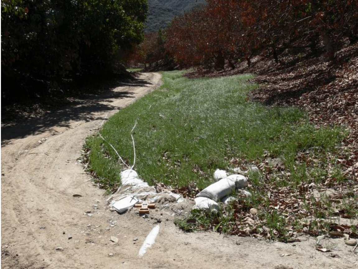
Drain B (photo 10): Looking south along the drainage from where it crosses under the access road (pipe partly exposed in the roadbed in the foreground). The tributary to this drainage connects about where the road bends in the distance. Conditions in the tributary are similar to those shown in photo8.
