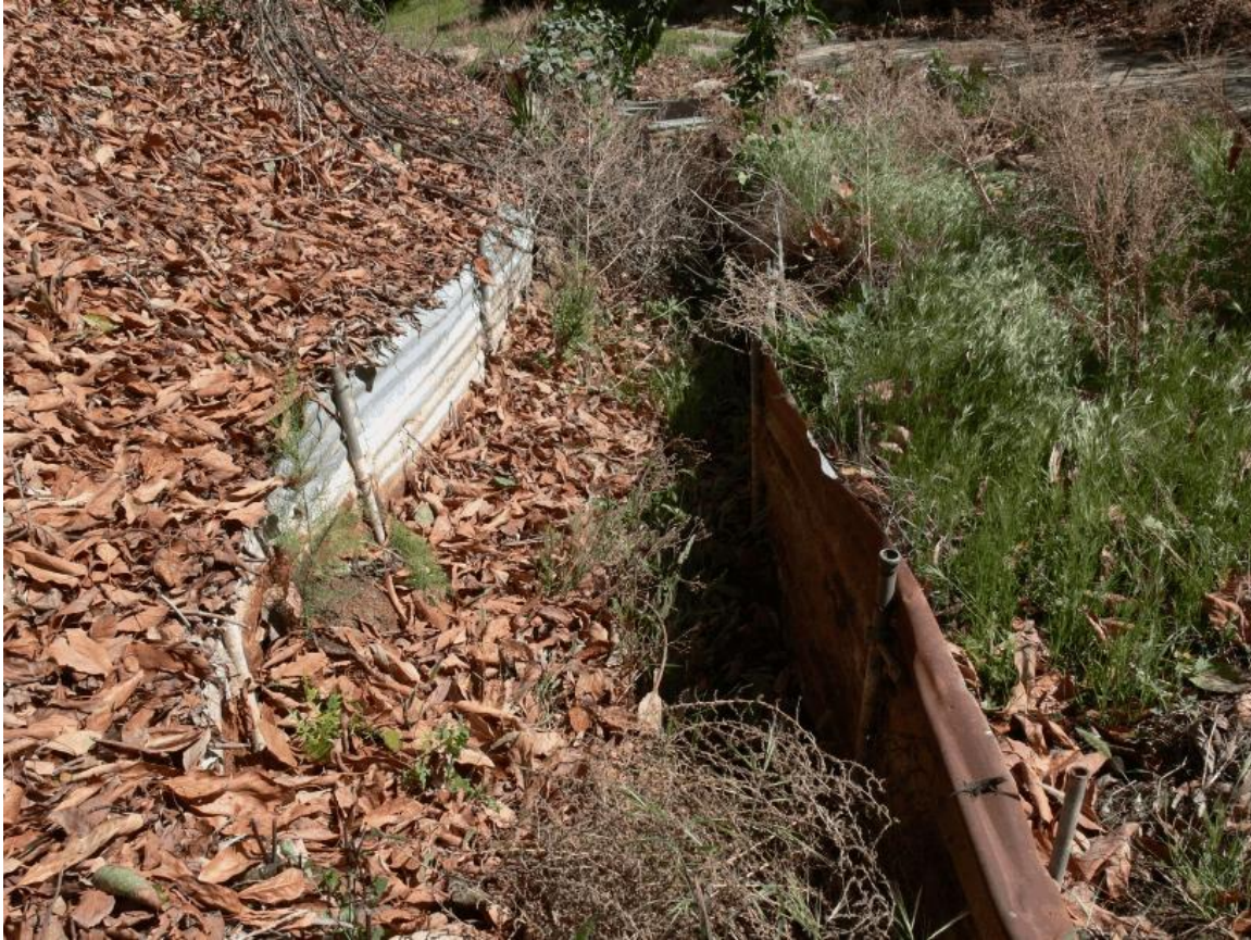
Drain A (photo 4): Looking north showing the metal corrugated sides of this part of the drainage and the high amount of leaf litter.
