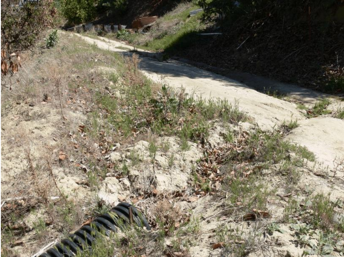
Drain A (photo 7): Pipe from previous photo empties into ditch along far side of this road, crosses the road, and empties into the pipe in the lower right corner of this photo.
