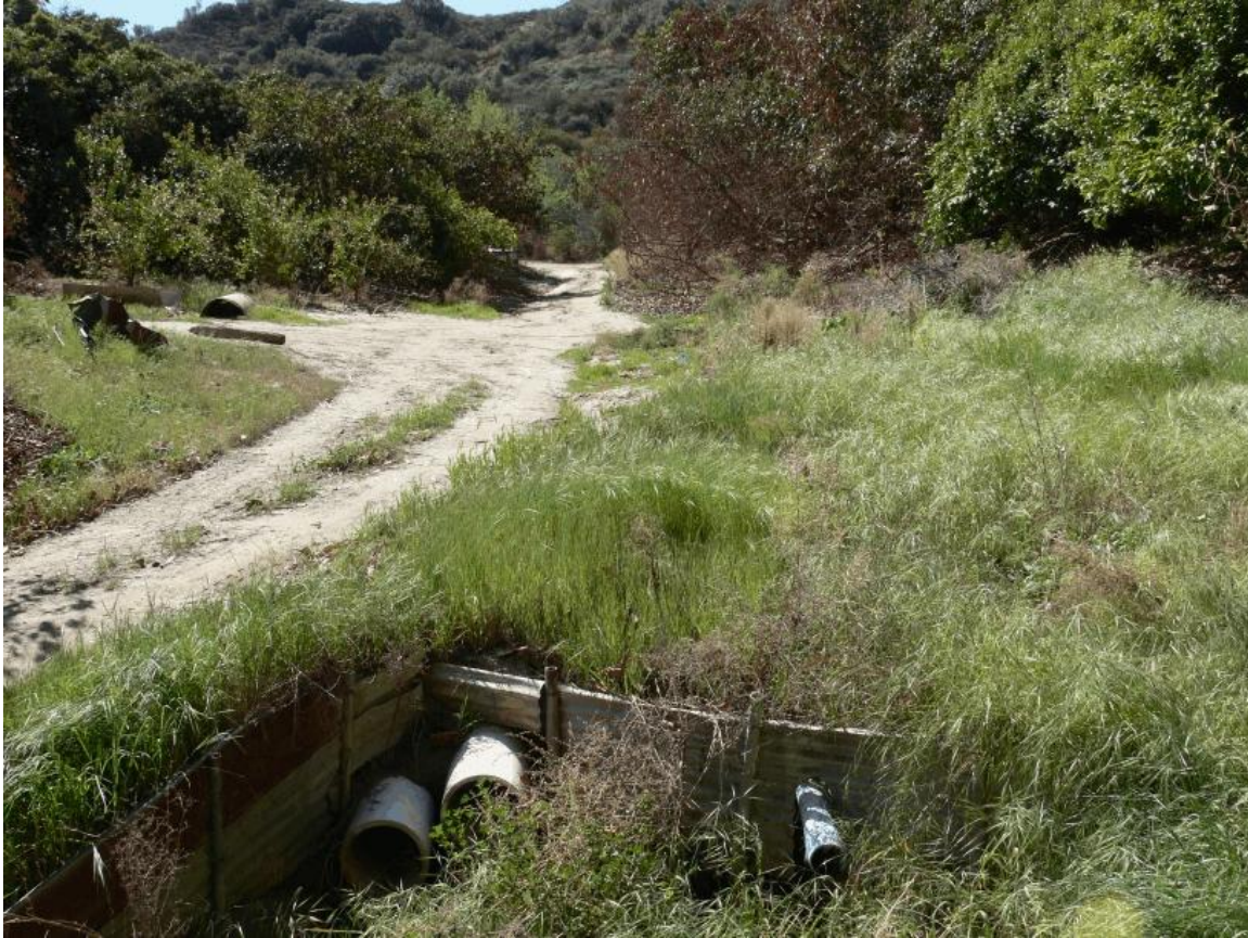
Drain A (photo 3): Looking south at point where pipes from willow tree daylight. Willow tree can just be made out at the end of the road in the distance.
