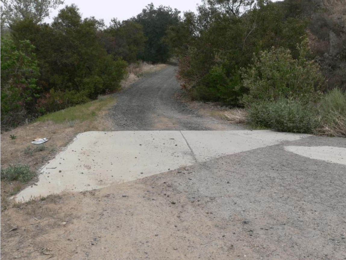
Drain E (photo 28): Looking northeast along the access road along the western edge of the project site. Drainage E passes under this road through a cement pipe from the bushes on the right side of the picture to those on the left side.
