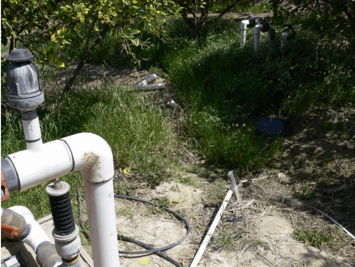
Drain D (photo 23): This photo shows the orchard water pump (left side of photo) and control valves (in the distance). The branch of Drain D nearest the main orchard access road can be seen passing between them. Water from the pump leaks into the drainage here.
