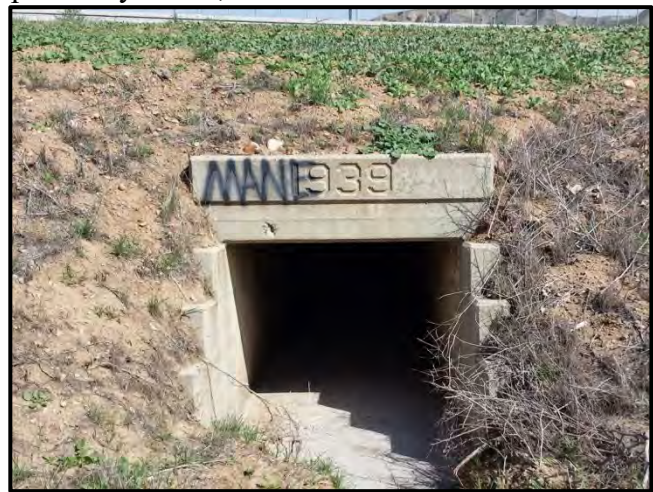
Plate 4.2–4: Circa 2014 photograph of what is likely the original 1939 culvert recorded by LSA in 2000. (Photograph courtesy of Ballard 2014)
