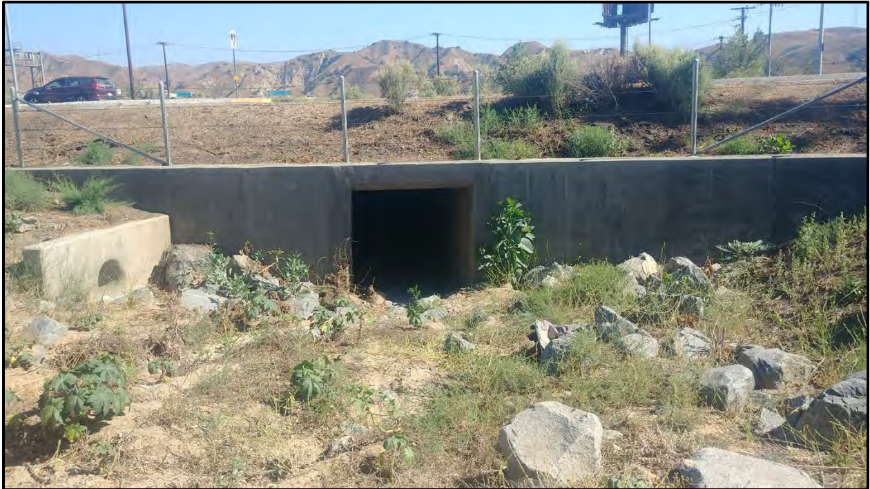
Plate 4.2–5: Overview of the new modern culvert within the project, likely installed during the Green River Road Widening Project, facing north.
