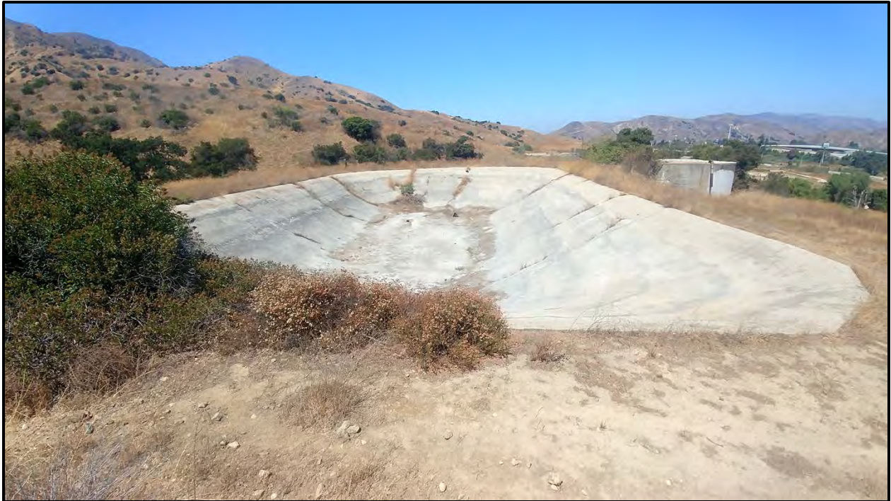
Plate 4.2–6: Overview of the concrete-lined reservoir and water tank at Site Temp-1, facing west.
