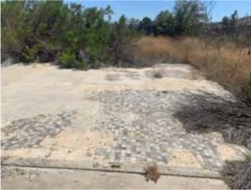
5. View east near northeast portion of the Site. Shows building pad condition.
