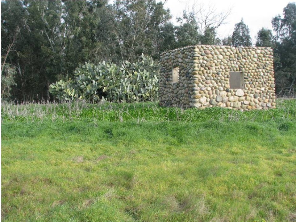
Photograph 12: Structural remnant of CA-RIV-1044. Reach IV and alternatives pass by this structure remnant, leaving it vulnerable to future vandalism.
